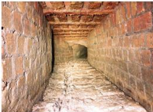
Section through the brick culvert connecting the sandstone tunnels through Church Aston Village
