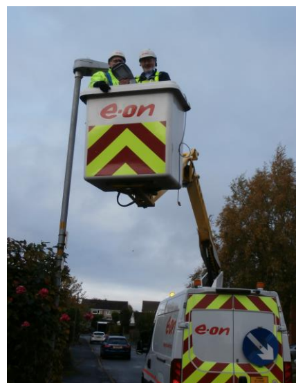
Cllr Brian Richards with EON operative Mark Simmons installing the final LED light at Mulberry Close
